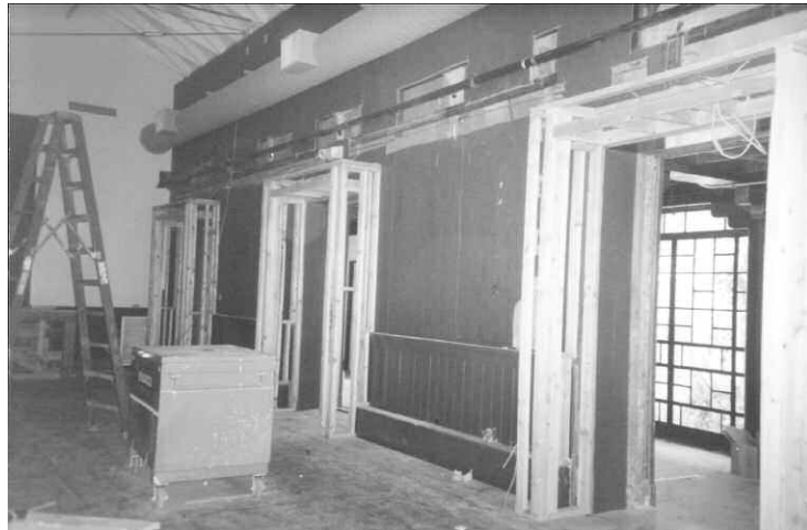
(Above) An Irene Poon Anderson photo documents the process of converting the gym of the 1932 Julia Morgan-designed Chinese YWCA into CHSA's main exhibit gallery. CHSA maintains the building as a city landmark. (Gift of Irene Poon Andersen, 2006.42.4)
